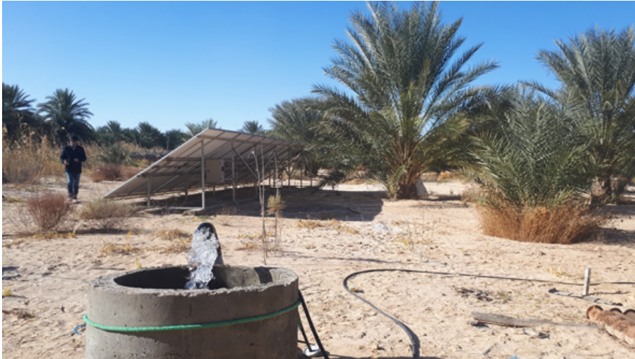
The irrigation system is operated with photovoltaic panels. The pump draws groundwater with energy generated by these panels.
